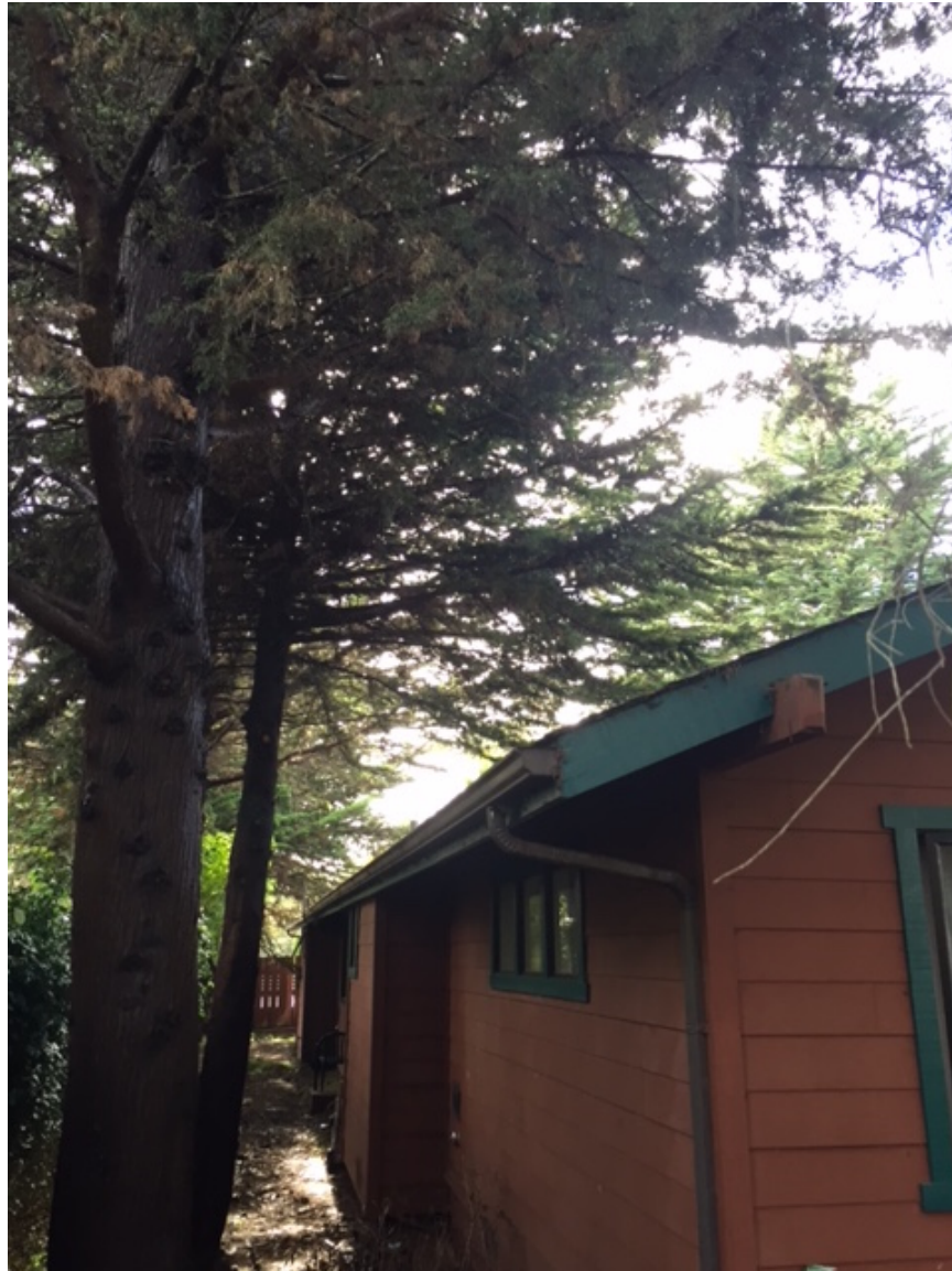
Figure 3. Additional canopy raising and trimming back limbs will be necessary for Cypress trees located behind building.
